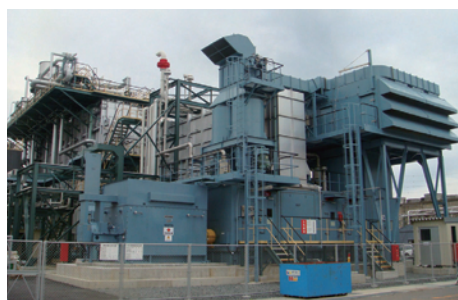
Cogeneration system installed at the Yokkaichi Plant.
